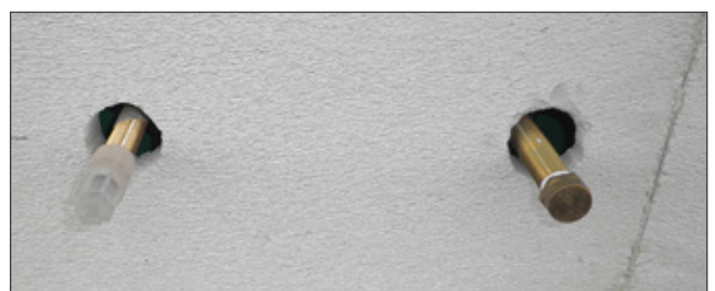
Fig. 3.3 – Neat finishes of installed services
