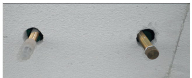
Fig. 3.3 – Neat finishes of installed services
